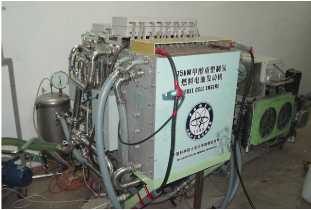
Fig. 3. Photograph of 75-kW fuel cell system.
